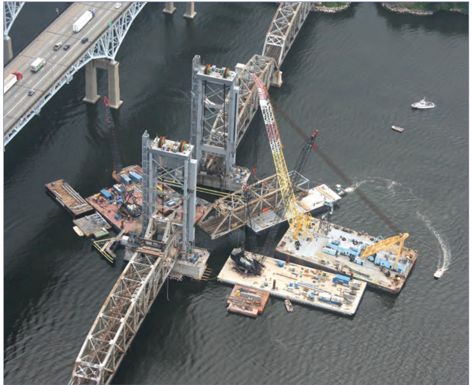
Donjon's heavy-lift equipment removes a span of an old Amtrak railroad bridge.
